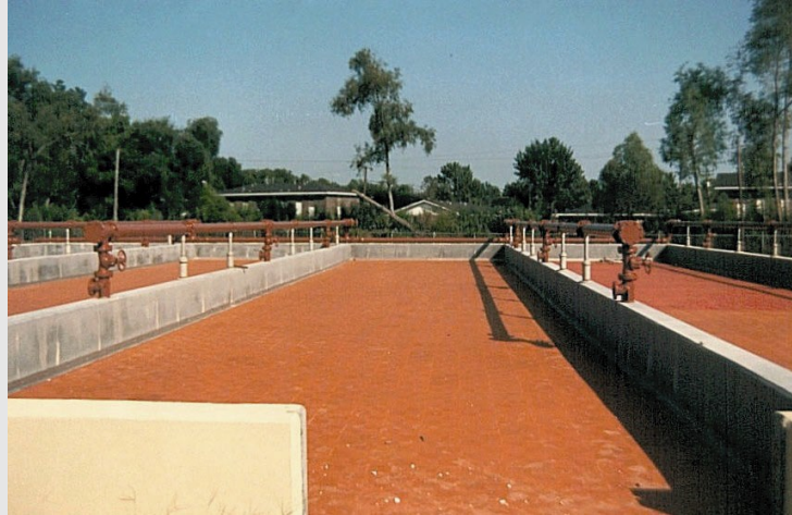
La Place, Louisiana Wastewater Treatment Plant — Four 1800 square foot Wedgewater™ Filter Beds
